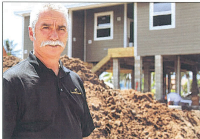
David Gydos of Tundra Homes is currently constructing a green home in St. James City.
